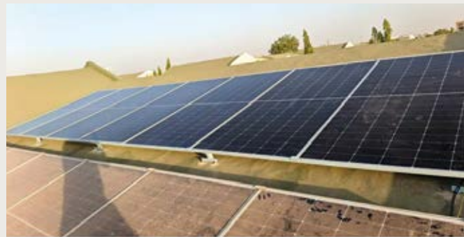
OHCHR-Ouagadougou 11KVA solar panel system © OHCHR
